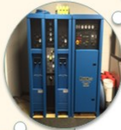
Breathing Air Compressor Replacement
